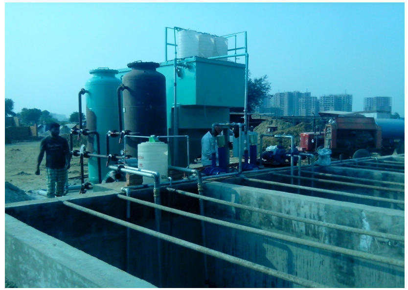
SEWAGE CUM EFFLUENT TREATMENT PLANT
