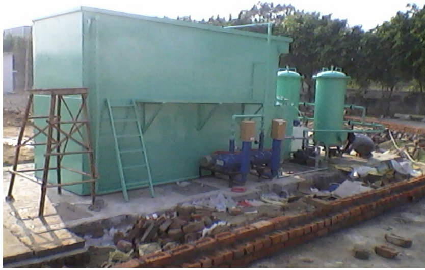
SEWAGE TREATMENT PLANT
