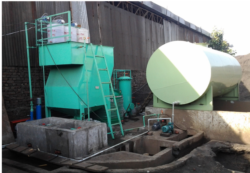
EFFLUENT TREATMENT PLANT
