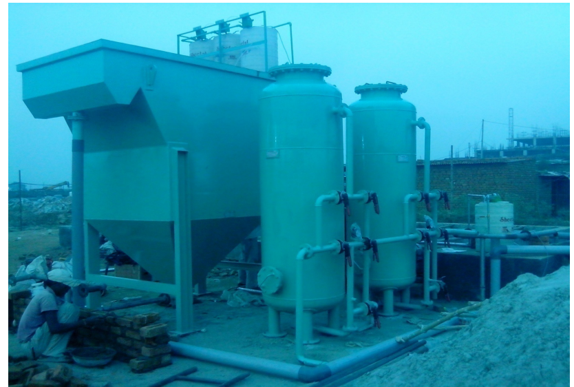
GREY WATER TREATMENT PLANT
